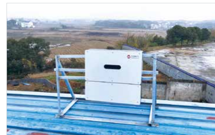
Rooftop PV Project in Hunan, China
