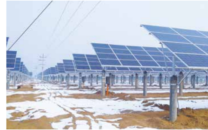
Poverty Alleviation PV Project in Hebei, China
