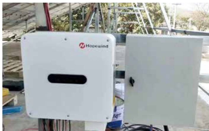
Residential PV Project in China
