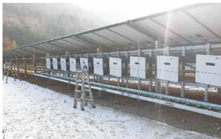
550kW Solar Plant in South Korea
