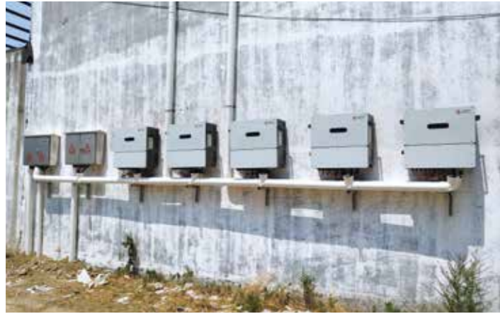
Rooftop PV Project in Shandong, China
