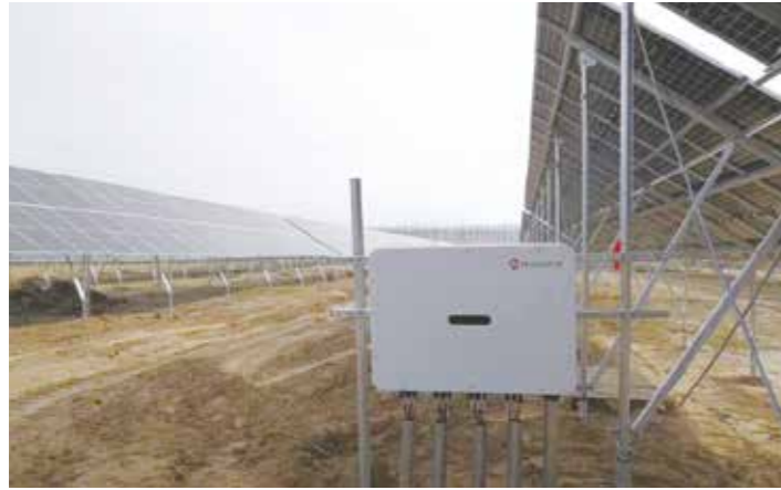
200MW hopeSunHV250KTL Utility Project in Ningxia, China
